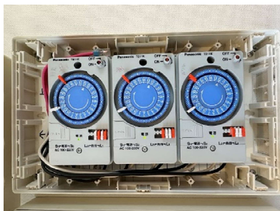
Timers in an electrical panel
